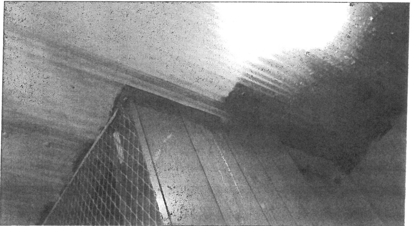
Photo #10 – No evidence of separation or movement of the roof panels above the wall that was displaced inward.
