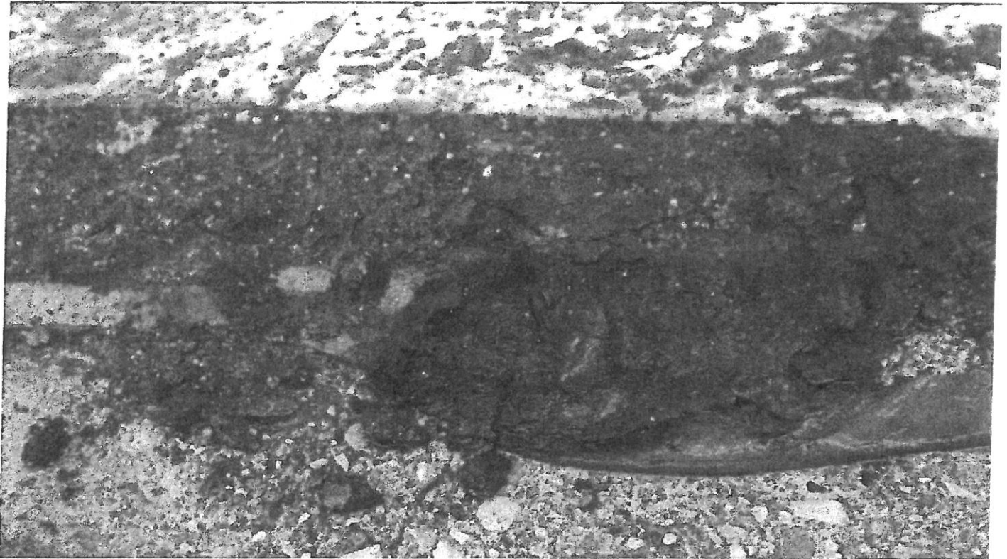
Photo #7 – The foundation anchor has corroded through.
