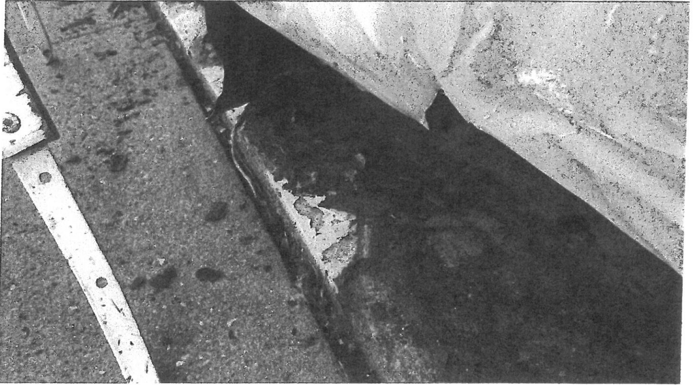
Photo #5 – The footing channel has corroded as a result of long-term exposure to moisture.
