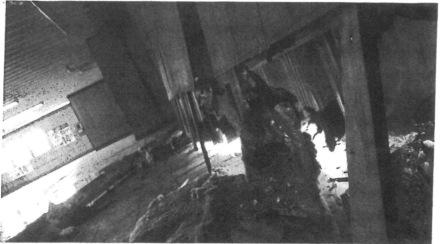
Photo #11 – View of the profile of the wall with furring and insulation.
